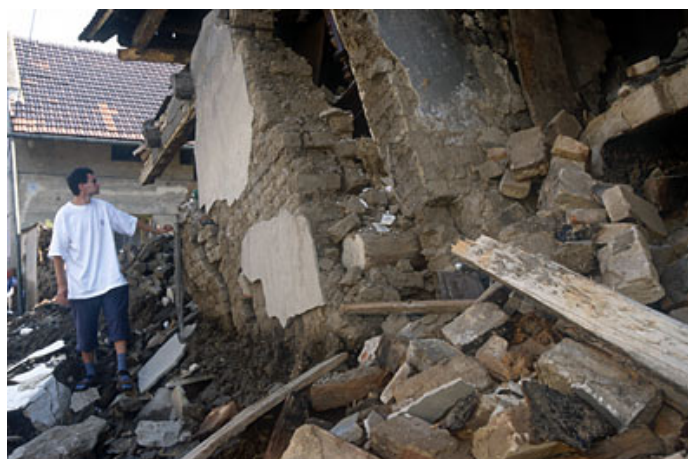
Traditional mud-brick dwellings collapsed in villages in North Bohemia, Czech Republic, August 2002 Photo: Andrew MacColl. IFRC
